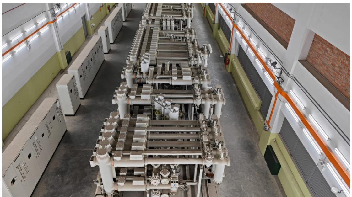
Kallang Basin 66kV substation
