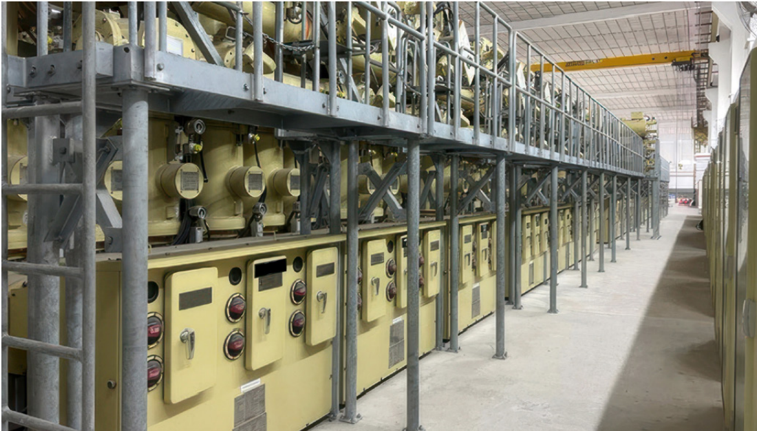
Paya Lebar 230kV substation
